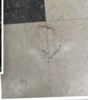
ABOVE: At 19 years old, the flooring at LBHS is well beyond its expected life and due for replacement.
